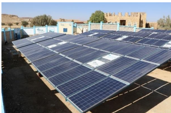
©UNICEF Yemen/2020. Solar panel water systems in Sa'ada.
