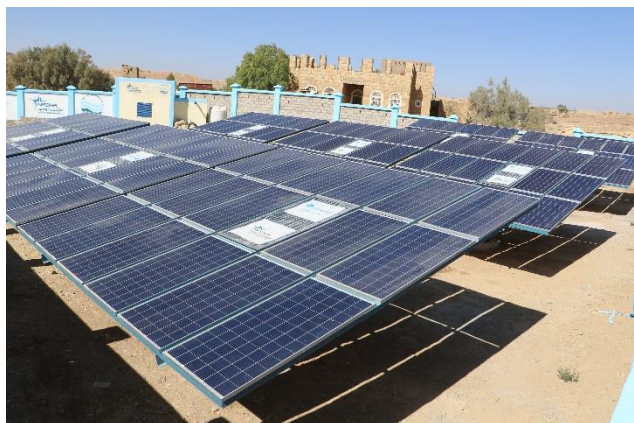
©UNICEF Yemen/2019. A rural solar project in Sada'a governorates.
