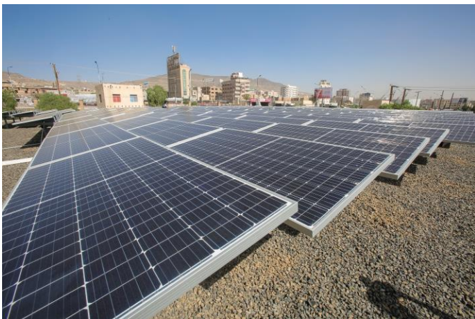
©UNICEF Yemen/2019/Majd Aljunaid. Solar panels have been installed inside a water plant to provide continuous access to safe water in a sustainable way to the inhabitants of Sana'a, with support of UNICEF and the World Bank.
