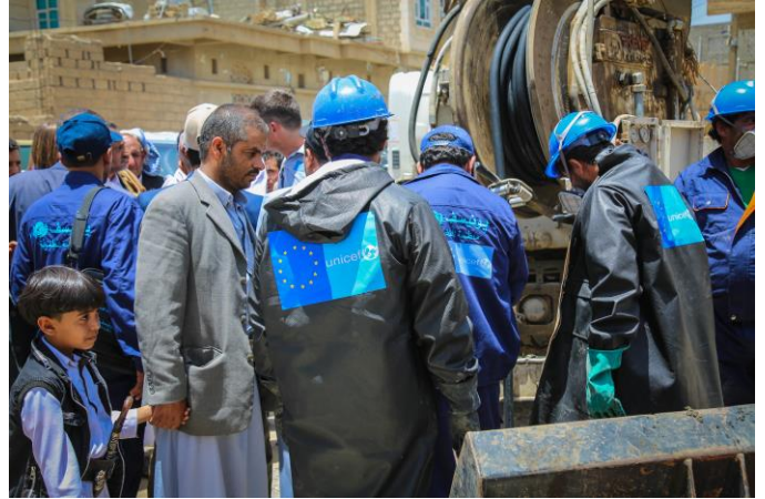
©UNICEF Yemen/2019/Ahmed Abdul Haleem. UNICEF WASH Team in Amran works hard to clean and rehabilitate the city's sewage network as part of the cholera response and thanks to the EU's contribution.
