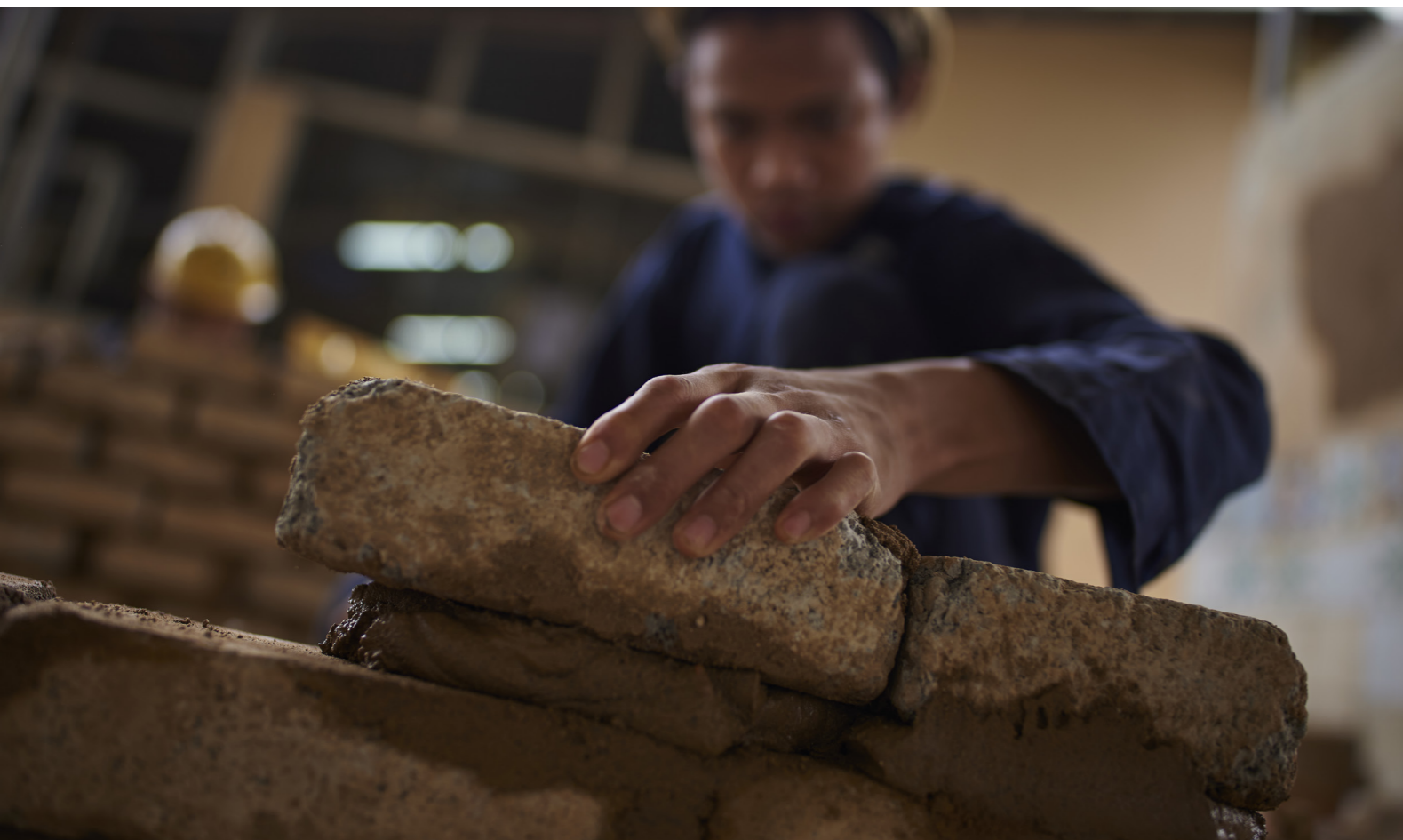
Akram (name changed) rebuilds a fallen wall inside the Henry Gurney School, a rehabilitation institution for juvenile offenders aged 14 to 21, in Keningau, Sabah, Malaysia. (2018) © UNICEF/UN0249963/Noorani
